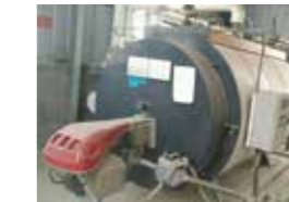
■ Air supply fan for boiler
