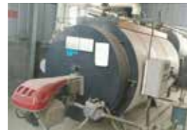
■ Air supply fan for boiler
