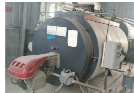
■ Air supply fan for boiler
