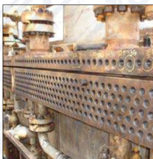
FinFan cooler before a maintenance
